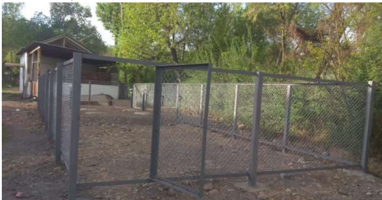
Figure 20. Example works on the subproject sites – Fence of the constructed septic tank
