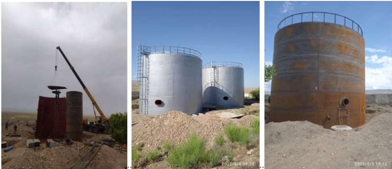
Figure 12. Example works on the subproject sites – Water tanks
