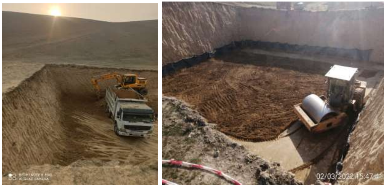
Figure 10: Example works on the subproject sites - Trench cross-section, depth of excavations, is regulated by the project
